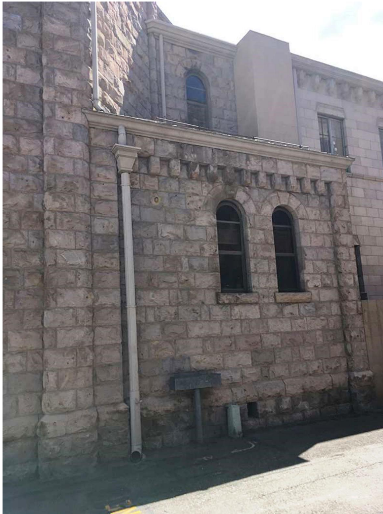
FIGURE 14.19 Panels W1 (two windows), W2 (singular window, above W1), part of W3 (to the left of W2), and W4 (left of drainpipe). This image shows the thick, dark, and continually present anthropogenic coating of Saint Elizabeth’s west facade. The coating extends the aspect’s entire length and about 1 m above ground level.
