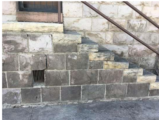
FIGURE 14.4 Panel N1, covered with a heavy (anthropogenic) coating. Notice also the missing mortarwork above the vent, creating a gaping fissure as well as other multiple cracks in the mortar.
