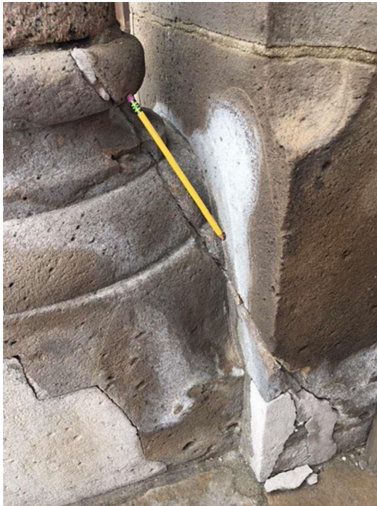
FIGURE 14.12 An example of fissures independent of stone lithification around column bases. This particular fissure (with a pencil for scale) occurs on E8. Just to the right of the pencil is a very light discoloration ( the white areas ) where salt efflorescence and subflorescence is occurring. Often occurring through capillary action, efflorescence, and subflorescence exert pressure on pore spaces, exacerbating interior vulnerabilities of the rock.
