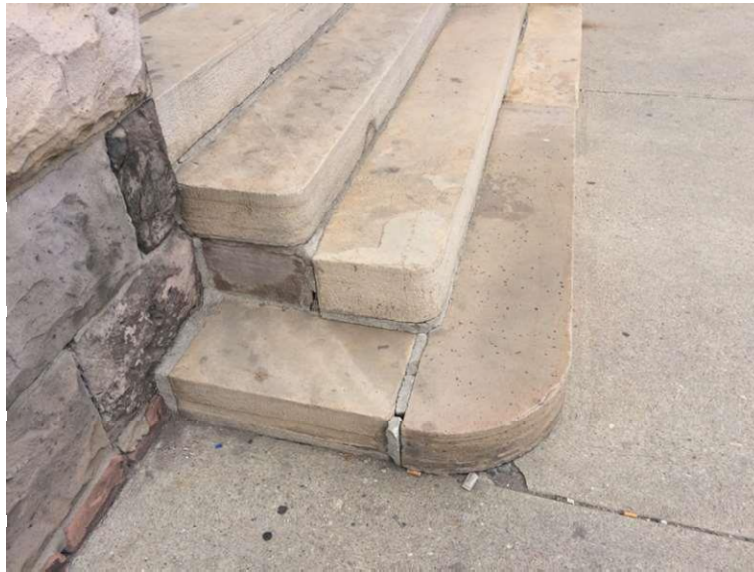
FIGURE 14.10 The stairs of Saint Elizabeth’s main entryway on the east-facing facade. As Saint Elizabeth is still a functioning church, it is no surprise that these stairs remain in “Urgent danger of erosion.” Specifically, notice the impending splintering of individual stairs and loose/cracked mortar, similar to N1 (compare Figs 14.4 and 14.5 ).
