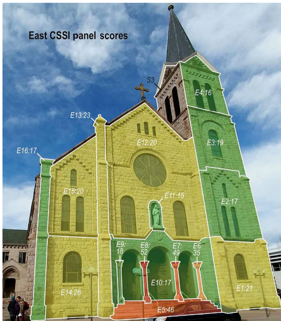
FIGURE 14.9 Saint Elizabeth's east-facing facade. Earning an overall score of 25 ("Good condition" status), the east facade has some looming problems that, if not addressed promptly, may result in large stone loss and the need for very costly repairs. In particular, E5, E7, and E8 remain at high risk, especially E7 and E8—the highest scoring panels on the entire structure and in "Urgent danger of erosion," specifically, at their bases (compare with Figs 14.13–14.16).
