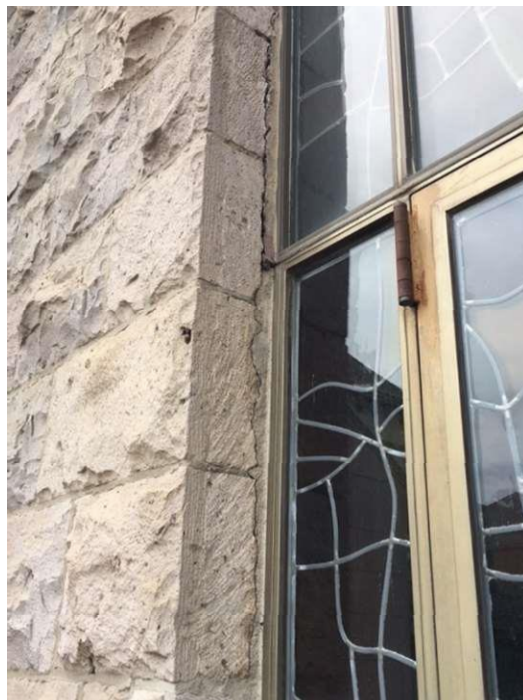
FIGURE 14.17 Creating similar conditions as seen on the underside of other window arches (compare Figs 14.10 and 14.17), the missing mortar along S1's window edge will ultimately lead to flaking and scaling events if left untreated. Specifically, note the large crack between the stone of the arch and the windowpane, extending from the old mortar work (bottom-center) all the way to the beginning of the curve of the archway.
