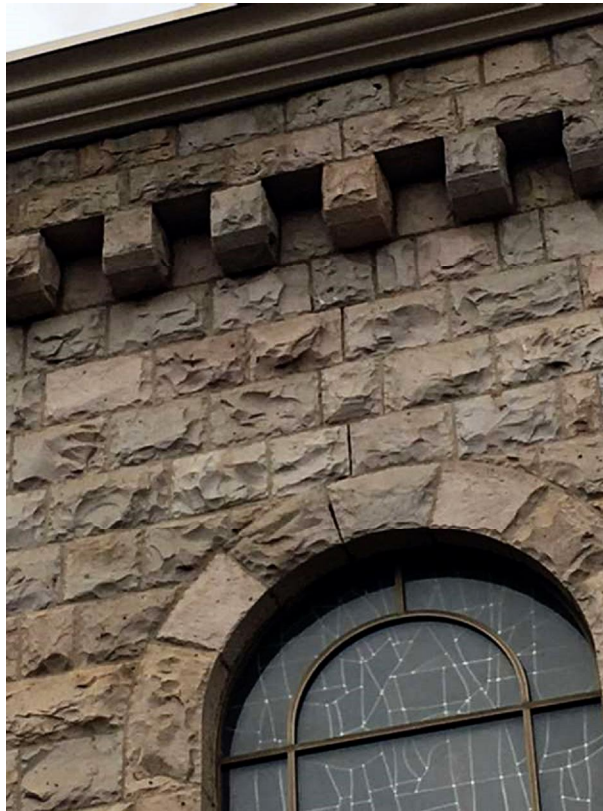
FIGURE 14.16 Beginning at the top of S2's highest window and extending across four bricks, missing mortar creates a gap in the masonry. The open space increases the probability of fissure formation and its resultant flaking and scaling events. This area remains perhaps the most at-risk section of S1.
